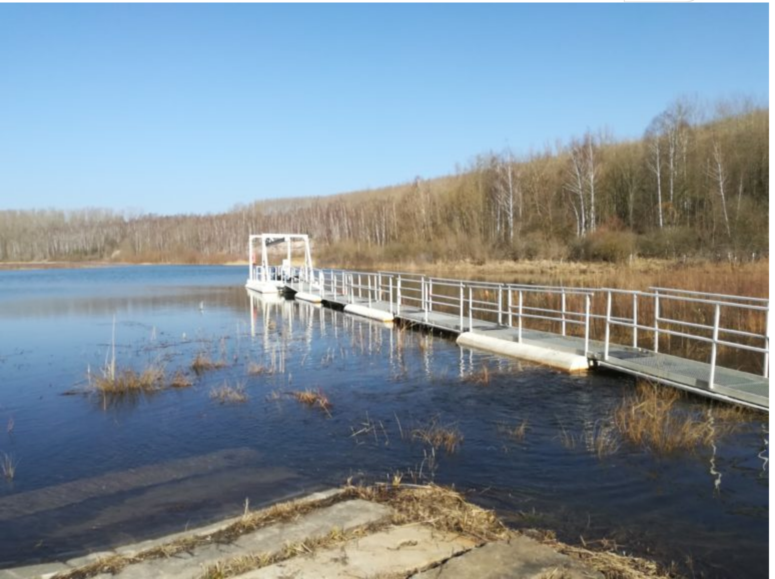
Pumpstation am Restloch Zechau III
